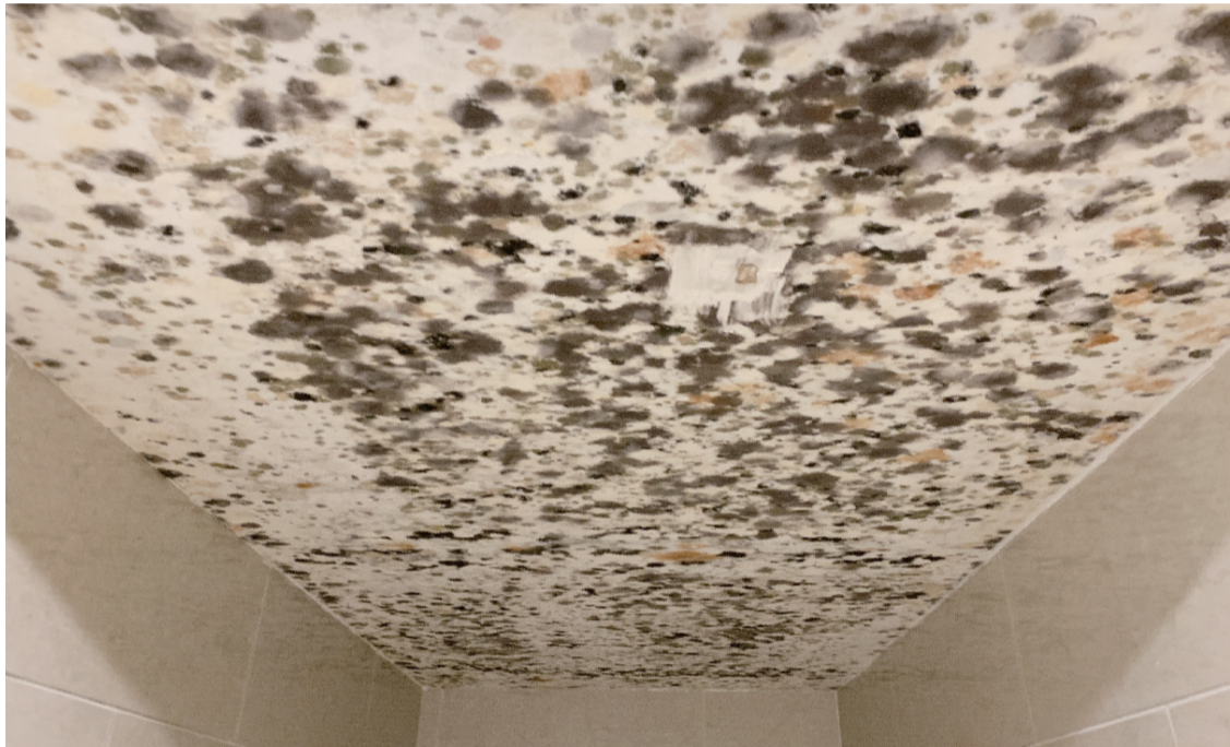
5号楼负二层楼板出现大面积发霉
